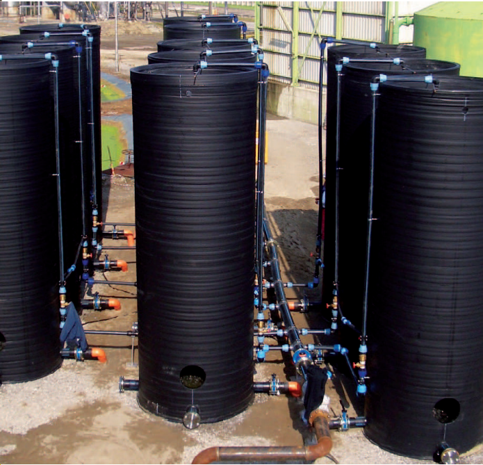
Landfill Collection Tanks
