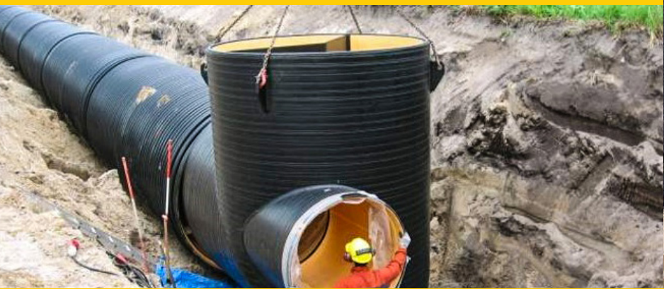
Stormwater Retention Tank
